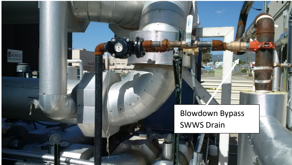
Photograph - NPDES-03A160-18-005 NHMFL Cooling Tower Blowdown Piping Connection to SWWS
