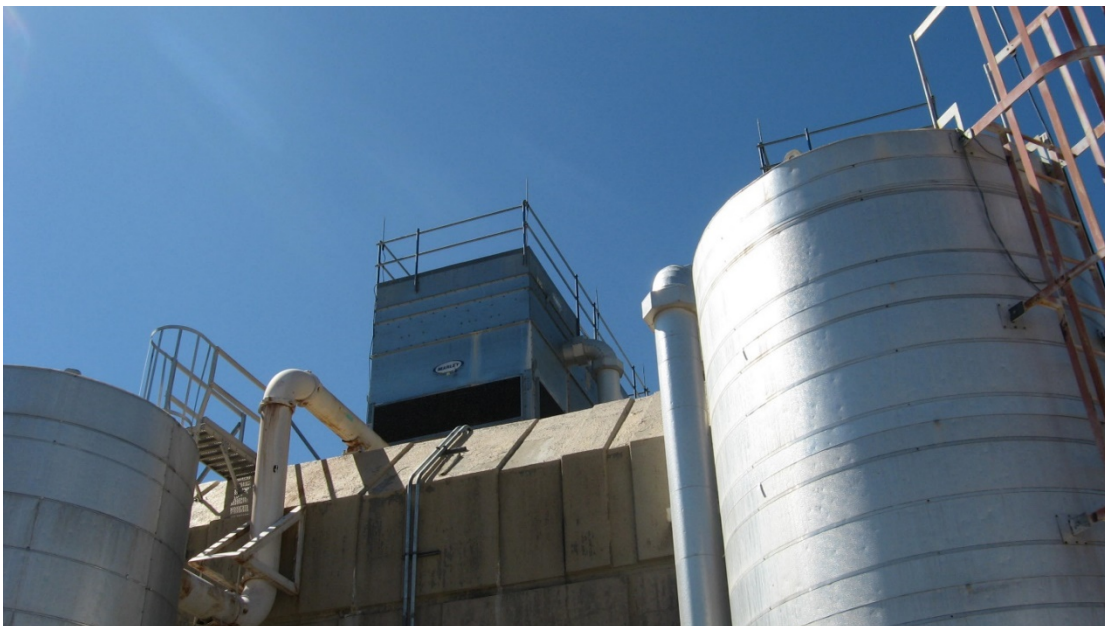
Photograph - NPDES-03A160-18-004 NHMFL Cooling Tower Holding Tanks
