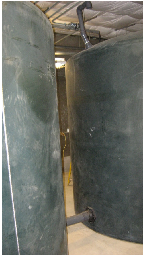
Photograph - NPDES-03A160-18-006 NHMFL Cooling Tower Blow Down Storage Tanks Prior to Discharge to Outfall 03A60 (inactive)
